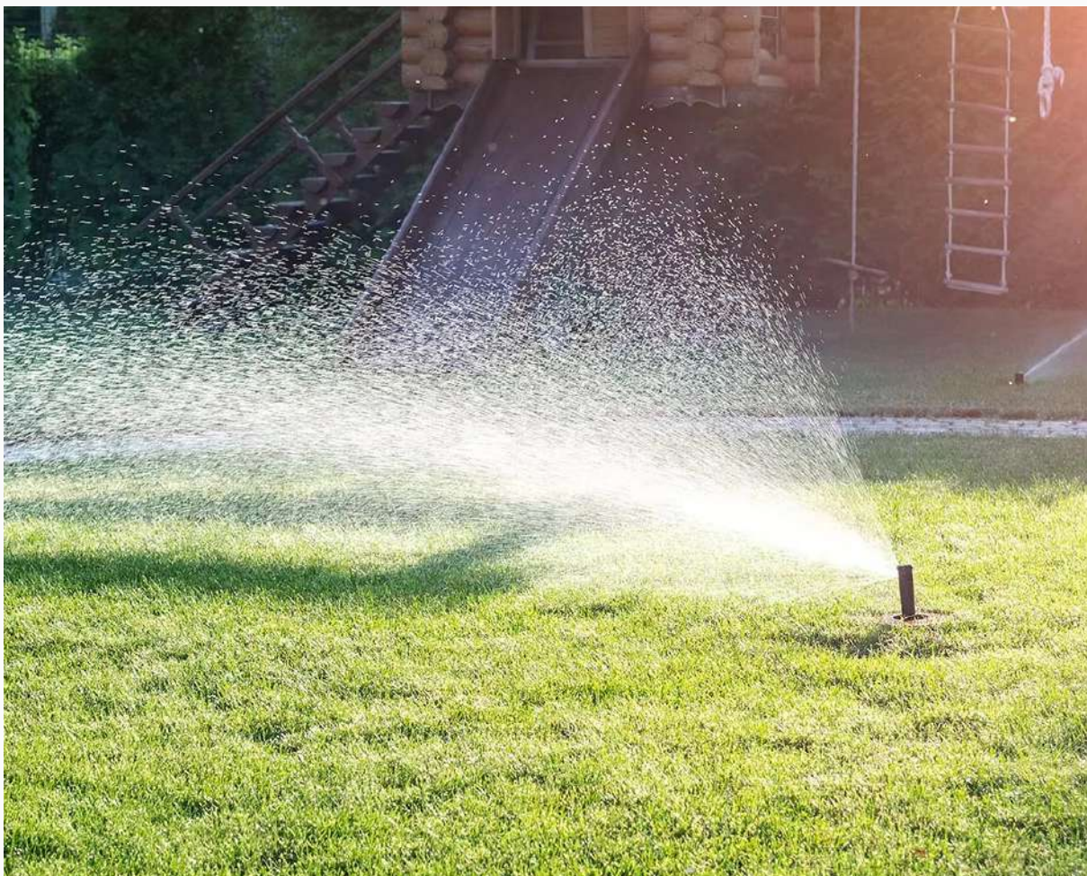
Lawn Automatic Irrigation
